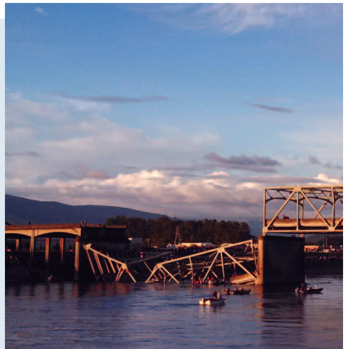
A section of Interstate 5 bridge over the Skagit River in Washington state collapsed after being struck by an over-height truck. While the bridge “was not considered structurally deficient” when it collapsed, it was still one of thousands of bridges carrying more vehicles and being used longer than intended.
